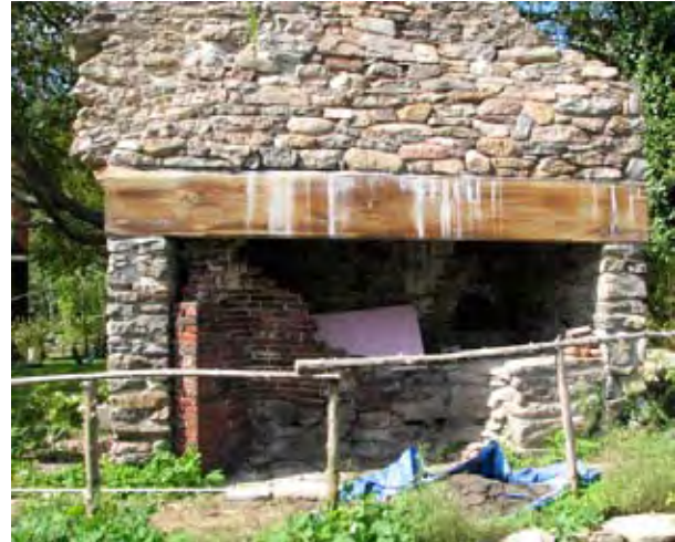
Figure 4.13: The current condition of the east side of the stone chimney with restored stonework and lintel and decaying later brick firebox, facing west.
