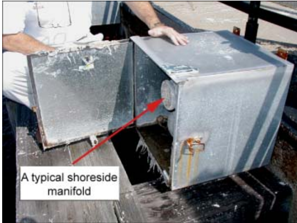
FIGURE 6. A typical shoreside manifold to which a large commercial vessel would connect its discharge hose and pump its effluent directly up and into a sewer line. The photograph is of the connector at Pier 4. Photograph: UHI
