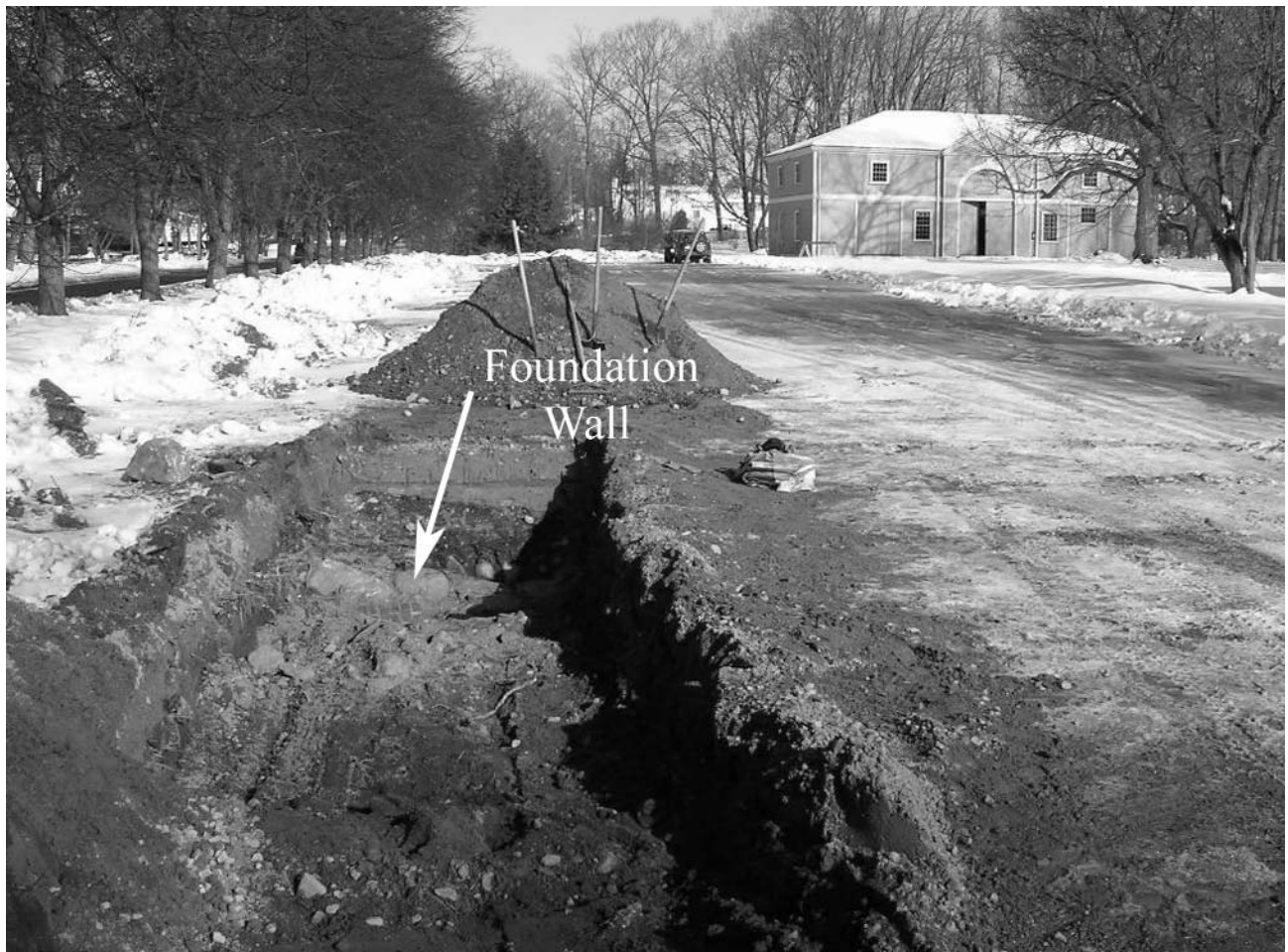
Figure IV.13. Carriage House Area Trench and Foundation Wall (facing north). Note post 1967 Carriage House location in background.
