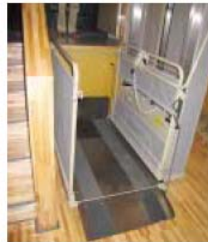
A lift installed in the gym
