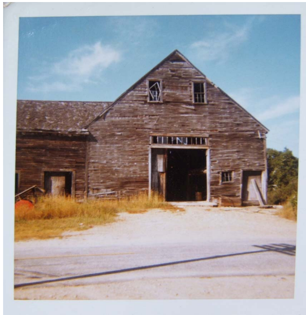
Figure 10: A 20 th century photo showing dilapidated state of the 19 th century barn.
