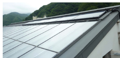
Heat collection panel (heat collection area: 507.4m 2 ) Photovoltaic power generation panel on the top row
