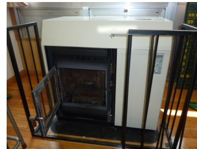
A pellet stove installed in a classroom
