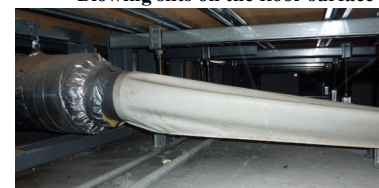
The duct under the floor of the gymnasium (Fabric duct: air blows evenly out of the fabric part)
