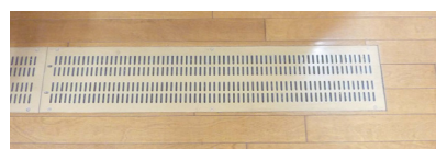
Outlet on the floor
