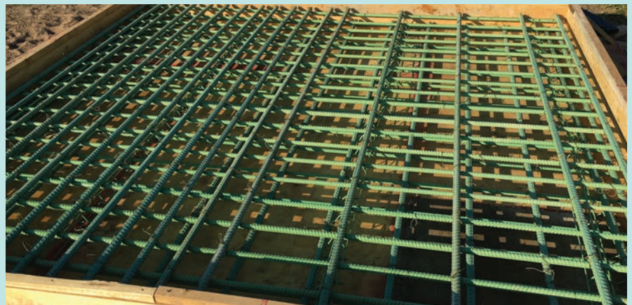
Mock-up slab placement with different top rebar spacing of 5x6 inches and 15x6 inches that correspond to different longitudinal rebar spacing locations along the bridge deck
