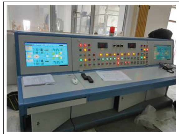
Figure 10. The automatic control system of coal mine main fans switchover.
