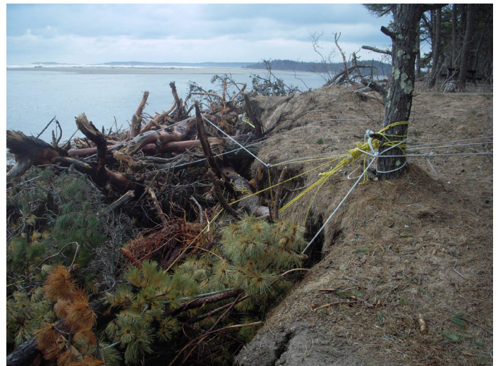
Figure 16a. Rafting of fallen trees to help stabilize the eroding bank along the bathhouse.
