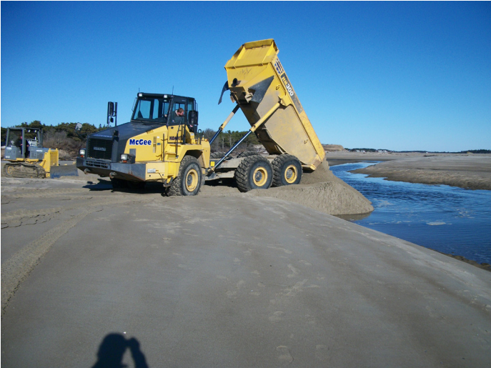
Figure 17a. Closing of the secondary channel in front of the bathhouse using beach scraping and mechanical equipment. Images by S. Dickson, MGS.
