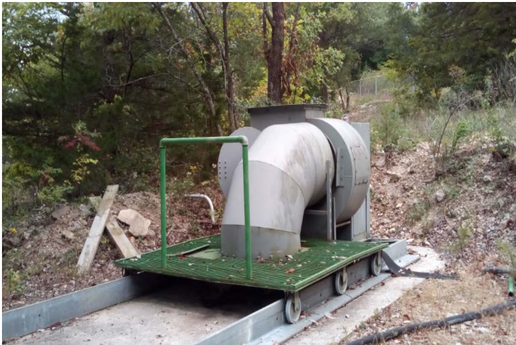
Figure 5.3. Illustration of exhaust fan at the surface
