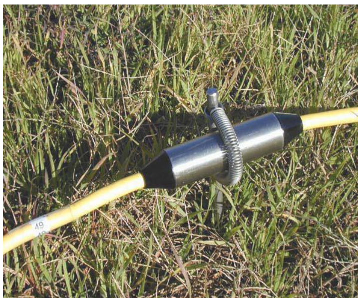
Figure 6.2. Electrode Switch Attached to the Stake
