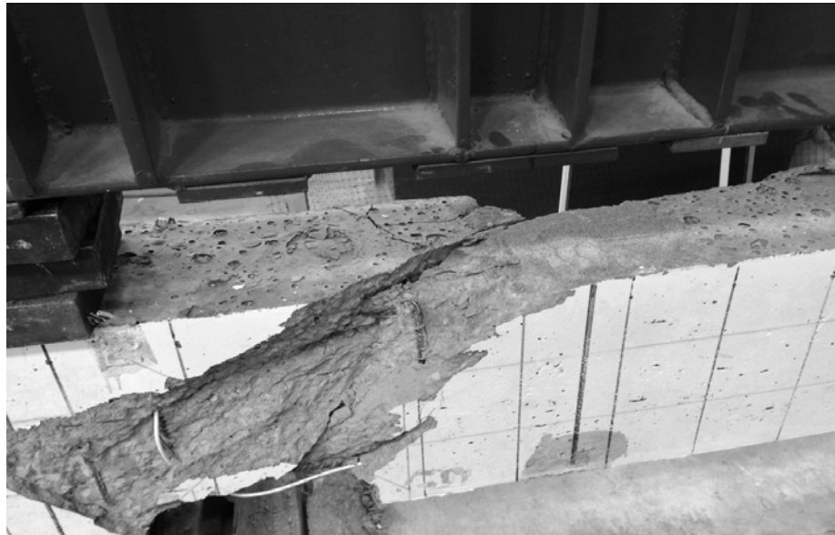
Fig. 12. Failure mode of GL6-2
