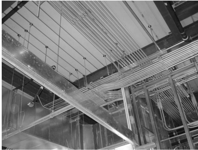
Fig. 1. MEP components suspended from steel roof deck
