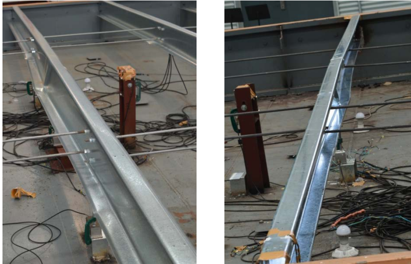
Figure 7. Failure modes of Z-purlin and C-purlin with two rows of sag rods
