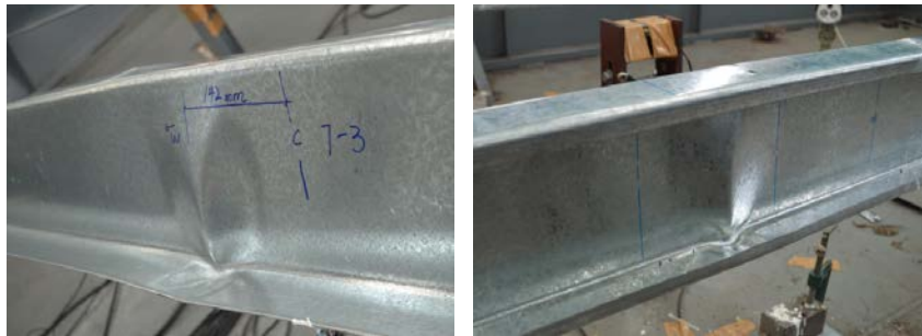
(b) Local buckling of Z-purlin and C-purlin
