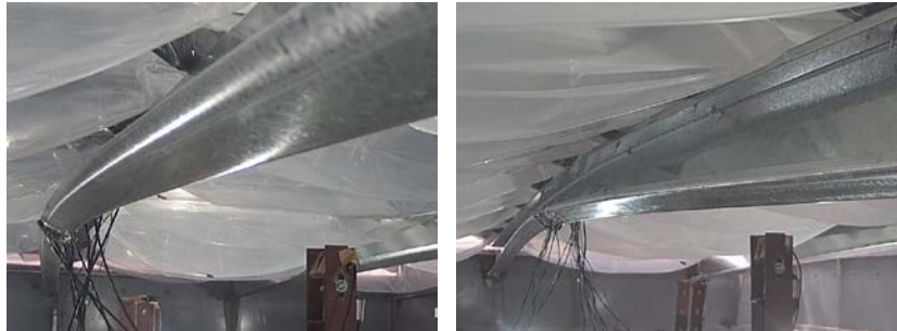
(a) Considerable lateral movement of Z-purlin and C-purlin
