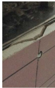
(e) gypsum board cracking
