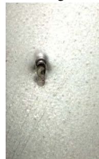
(f) steel sheathing bearing and tearing
