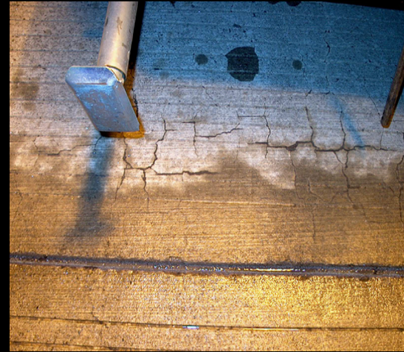
Cracking Near Joints
