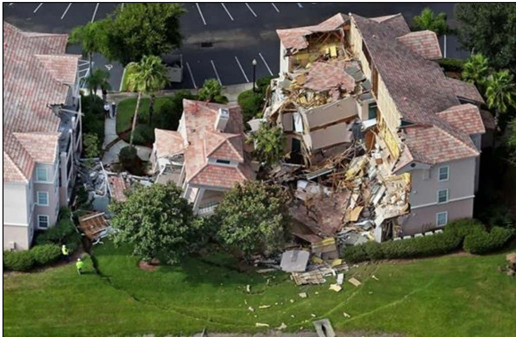
Figure 2.8. Buildings collapse into a sinkhole at the Summer Bay Resort in Clermont, Florida. ( http://www.amusingplanet.com/2013/09/disastrous-sinkholes ).
