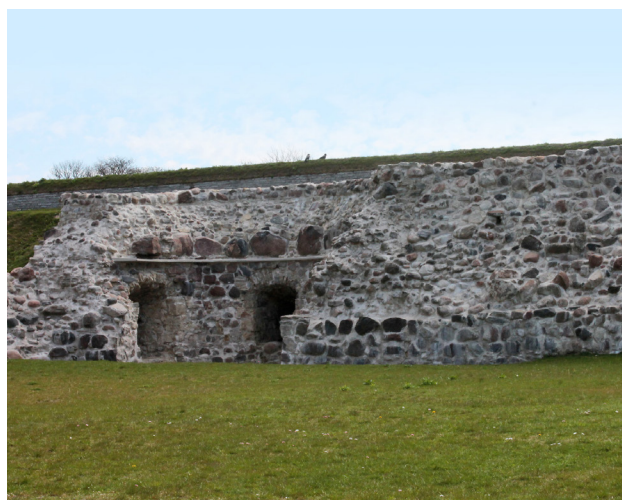
Fig. 12. The structure of the defensive wall of the castle in Kuressaare, photo J. Łach
