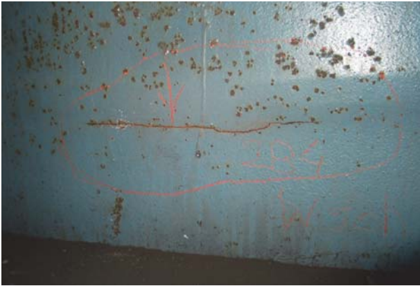
Fig. 5. Coating crack – 284 mm long – above the long support
