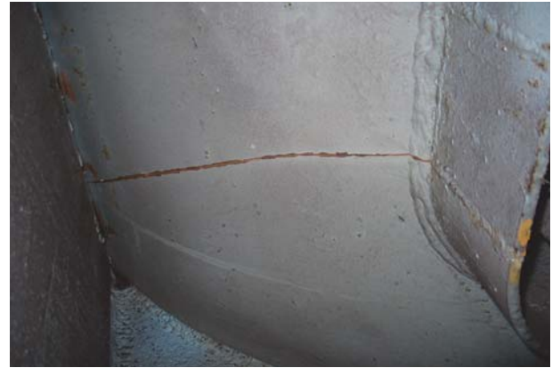
Fig. 6. Crack of the short support tube buffet – at app. 1/3 of a perimeter
