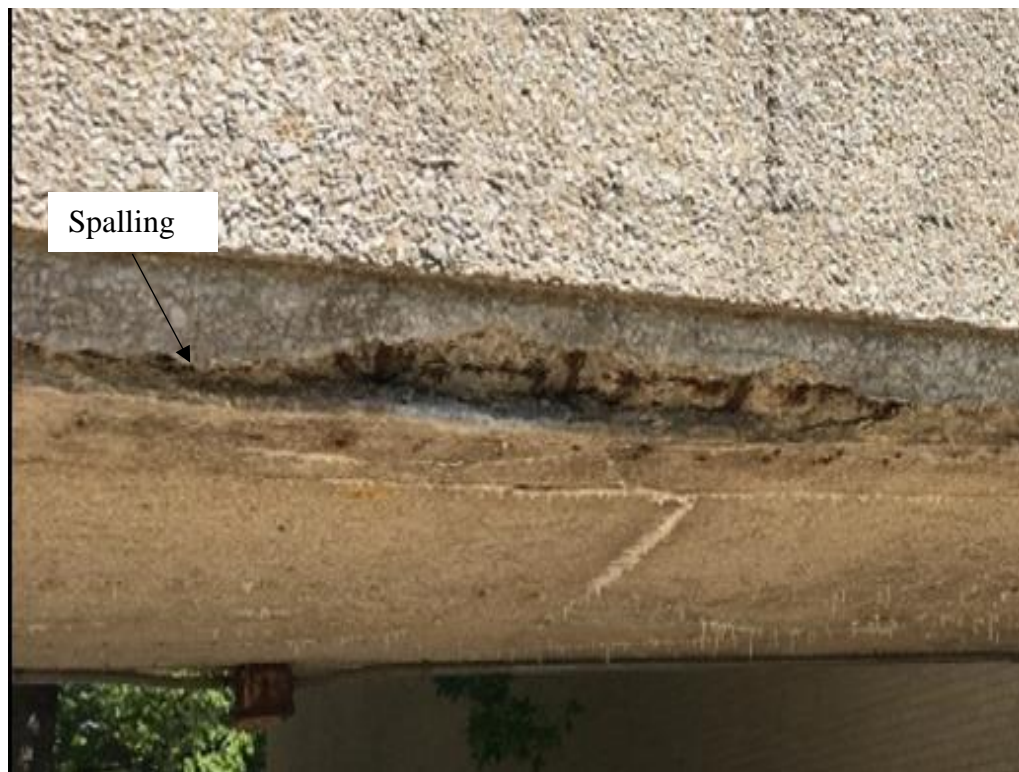
Figure 1.2. Bridge deck deterioration shows spalling.
