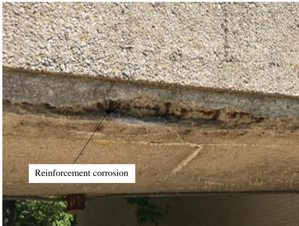
Figure 1.3. Bridge deck deterioration shows reinforcement corrosion.
