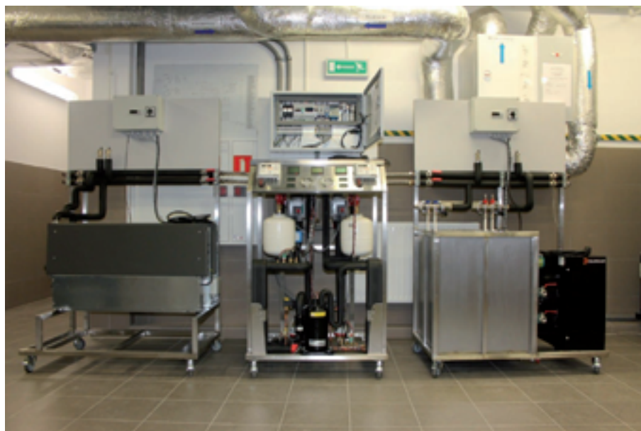
Fig. 3. Didactic air-water type heat pump. Energy source, heat pump and heating system modules
