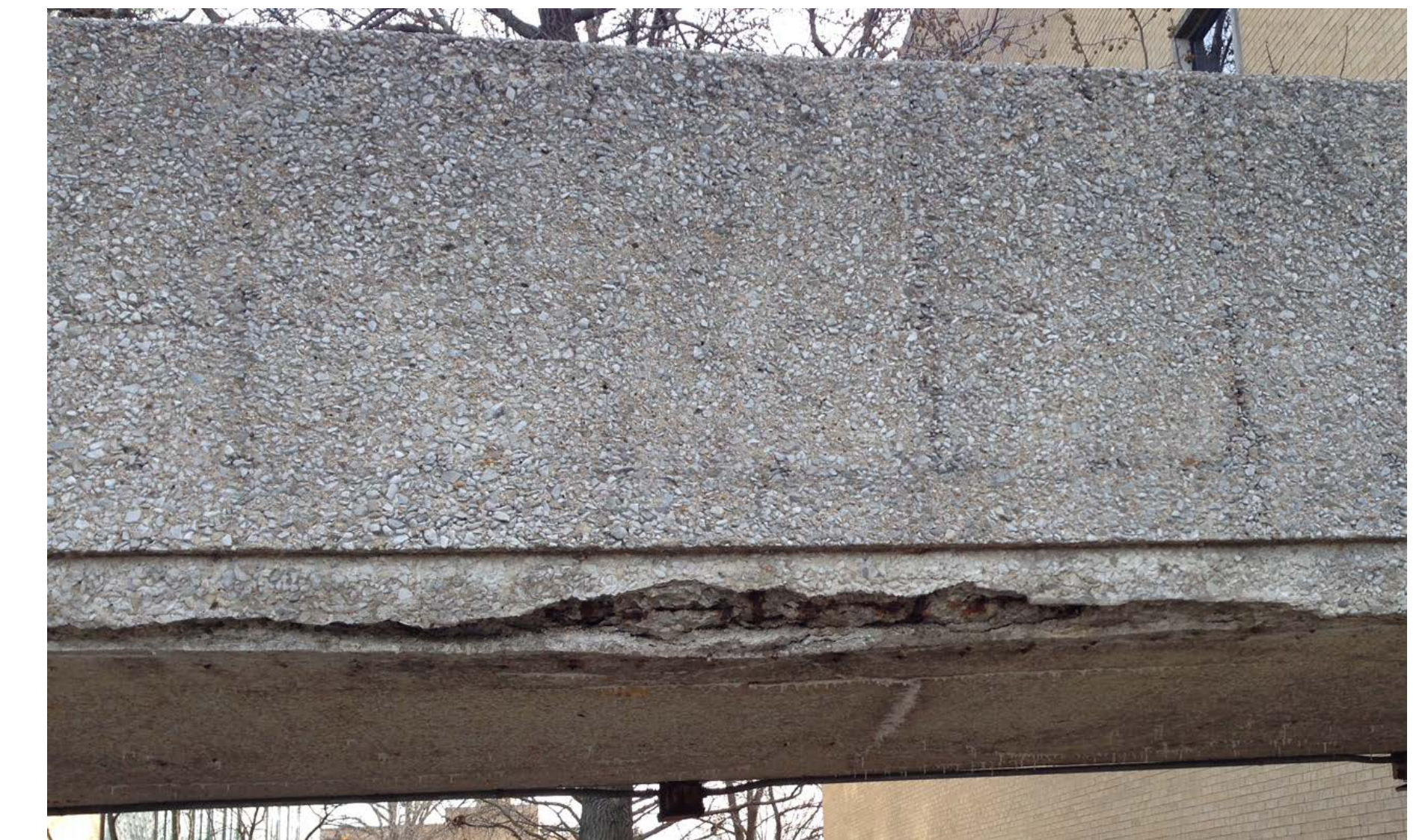
Figure 5: Pedestrian bridge with potential corroded rebars and delamination.
