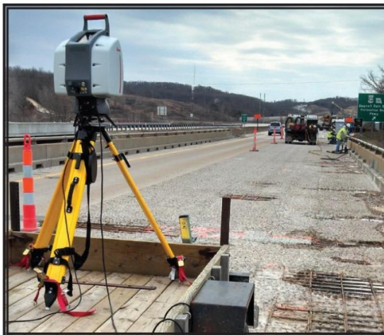
Fig. 5. LiDAR scanner set up to scan the bridge deck after hydrodemolition was used to remove unsound concrete.
