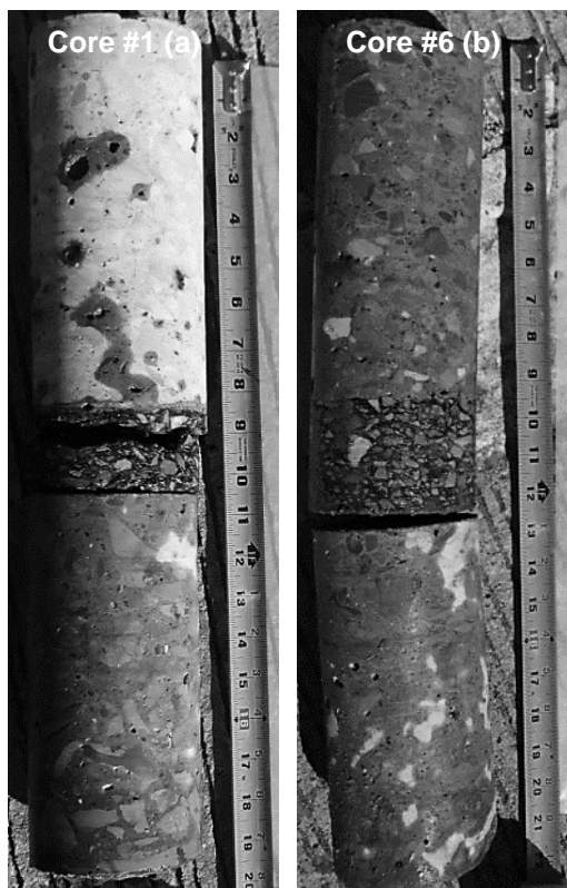
Figure 6. Photos of typical deteriorated (a) and intact (b) core specimens retrieved from experimental site.
