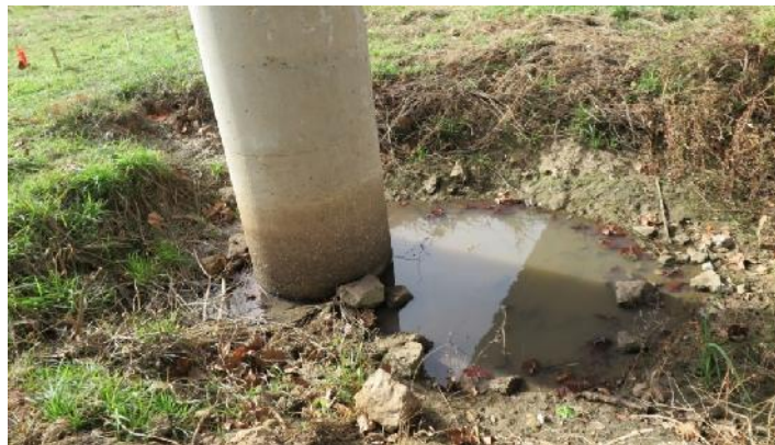
Figure 4.5. The bridge pier with a scour hole as a field test site.
