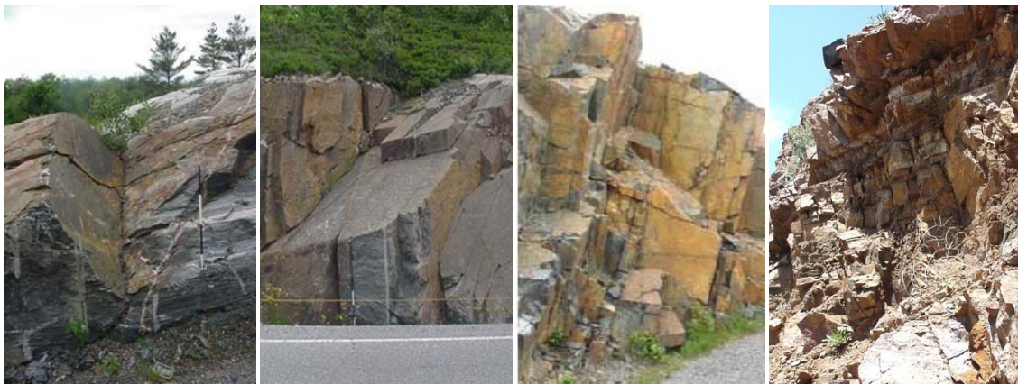
Figure 2.1. Example of Different Failures. Wedge (far left), Planar Sliding (middle left), Toppling (middle right), and Raveling (far right) (Maerz, 2012).
