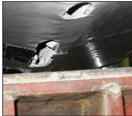
(c) Rupture of Polyurea
