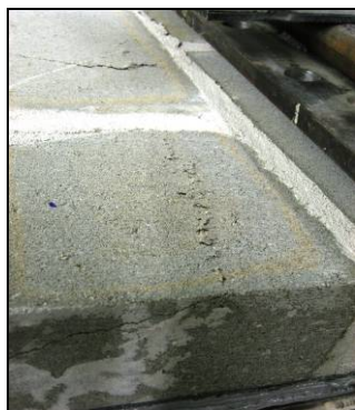
(a) Flexural-Shear Cracks
