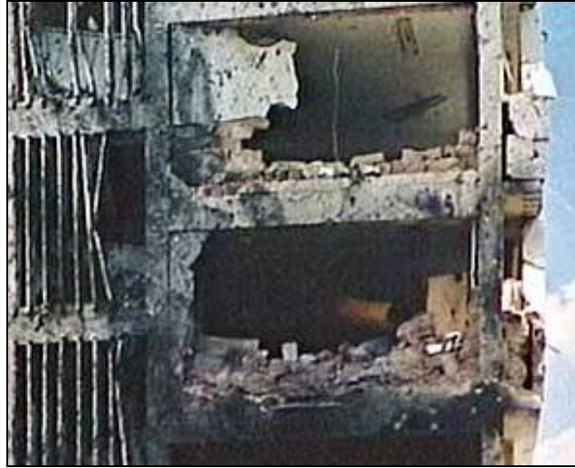
Figure 1.2. Failure of Exterior URM Infill Walls
