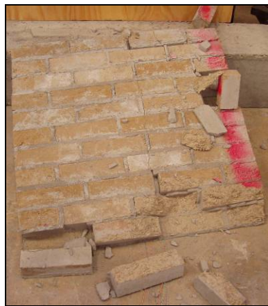
(a) Wall Collapse
