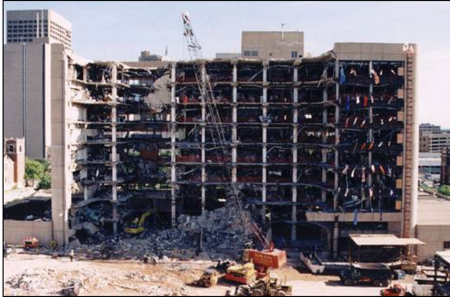
Figure 1.1. Damage to Alfred P. Murrah Building (FEMA, 2003)
