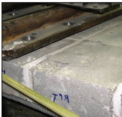
(a) Masonry Rupture
