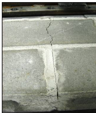
(b) Longitudinal Cracking
