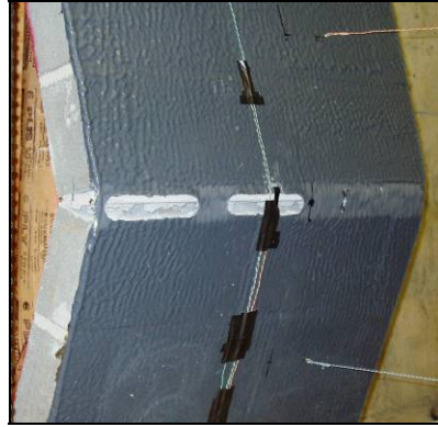
(b) Rupture of Polyurea
