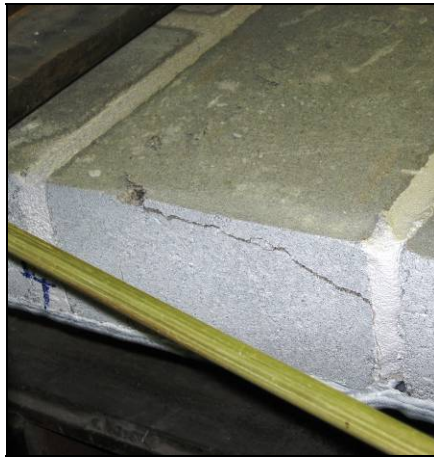
(a) Flexural-Shear Cracking
