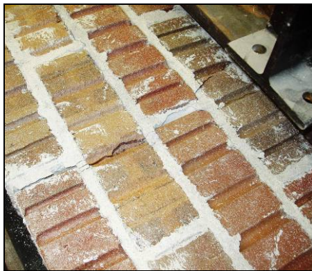
(a) Longitudinal Cracking
