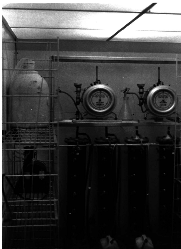
Figure 4. Anaerobic Filters and Feed System, Housed in an Environmental Chamber
