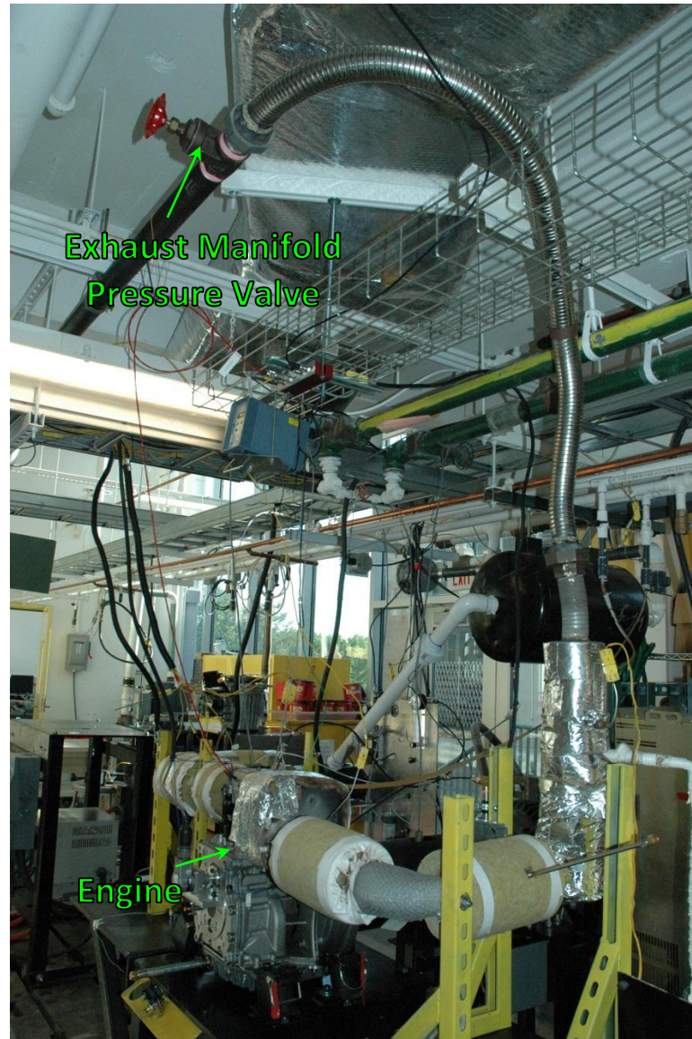
Figure 3.4. Exhaust piping – exhaust manifold back pressure valve
