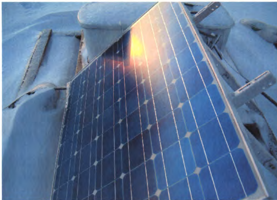
Figure 2.6. Solar Panel after Ice Melted Off, the Day after the Storm
