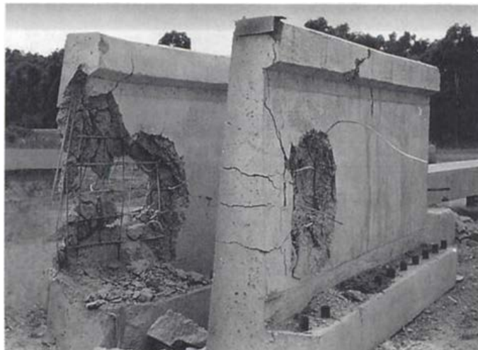
Figure 1.1: Reinforced concrete after EFP impact.(2)
