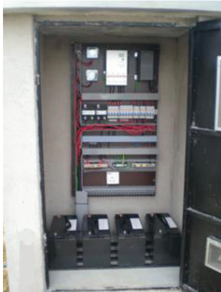
FIGURE 7 Housing for Batteries and Balance-of-system Components
