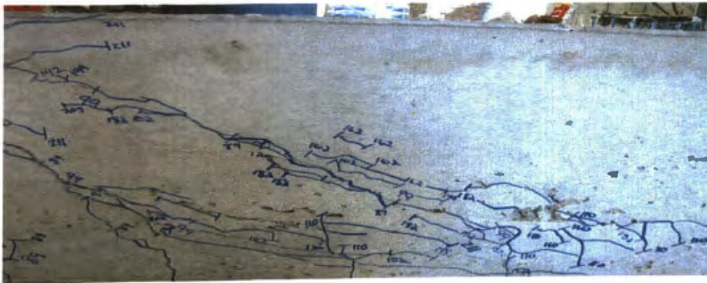
Figure 6.56. SCC-7-2 Beam at Failure
