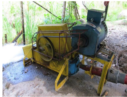
Figure 1: A MHEP system at a remote village in Sarawak [9].
