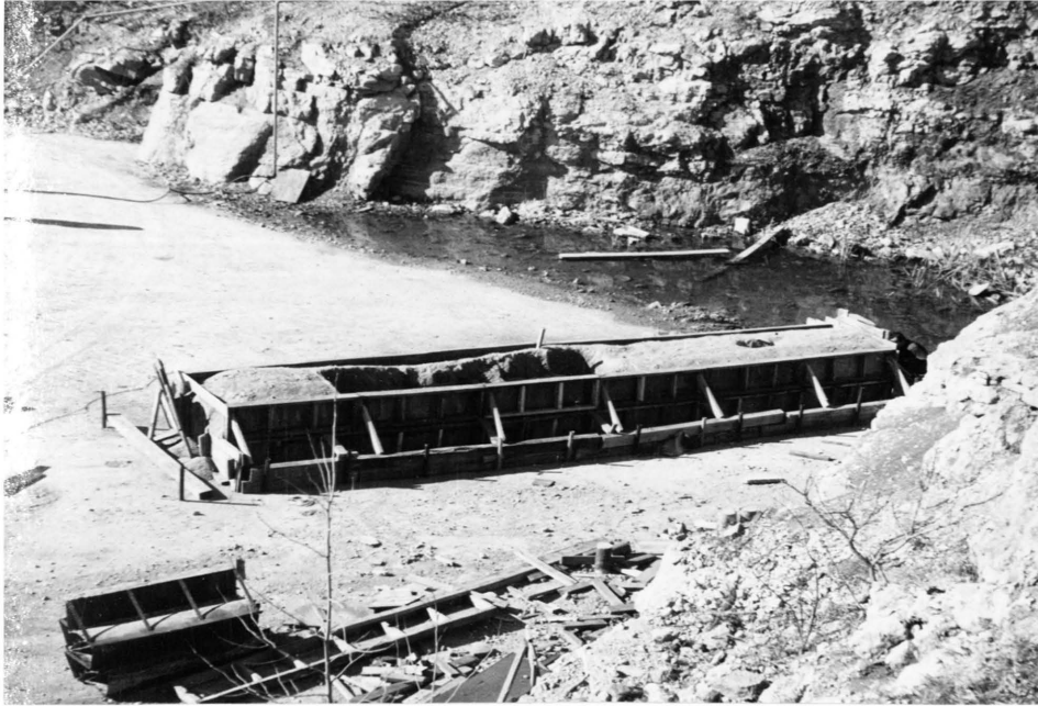
Figure 64. The results of the damage in Phase VIII.
