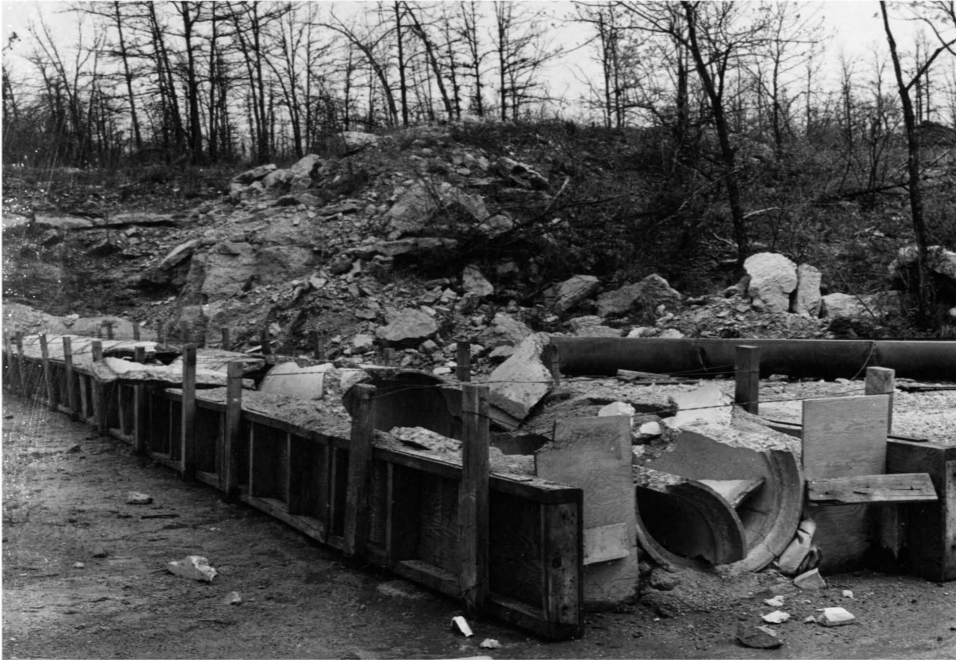
Figure 66. The damage resulting after demolition in Test Two, Phase IX.
