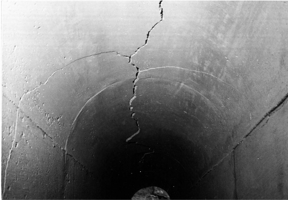
Figure 38. The results of demolition in Test Six "A", Phase II. The picture taken from the west portal.
