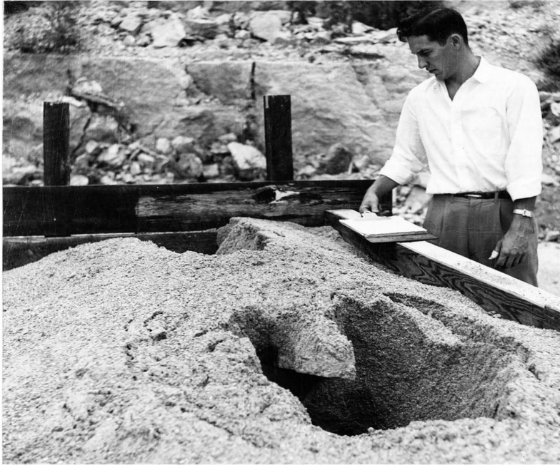
Figure 43. The results of the secondary demolition in Test Seven "B", Phase II.
