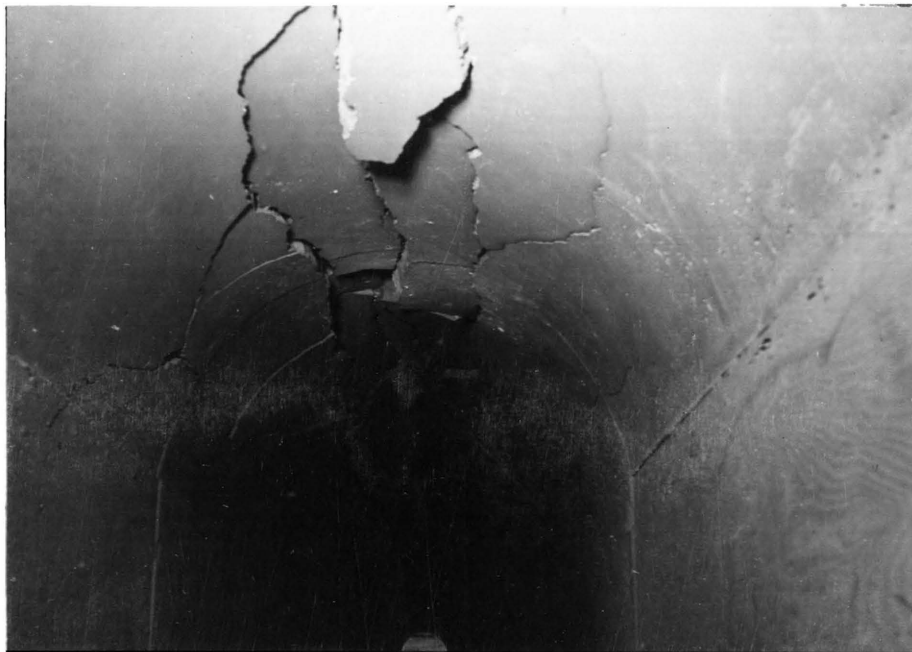
Figure 41. The results of demolition in Test Seven "A", Phase II. The picture was taken from the west portal.
