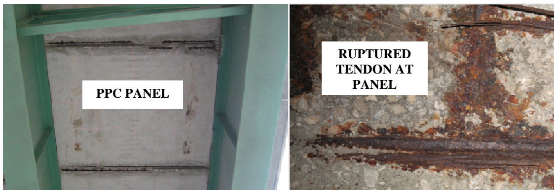
Figure 1.2. Spalled sections of concrete at various panel joints
