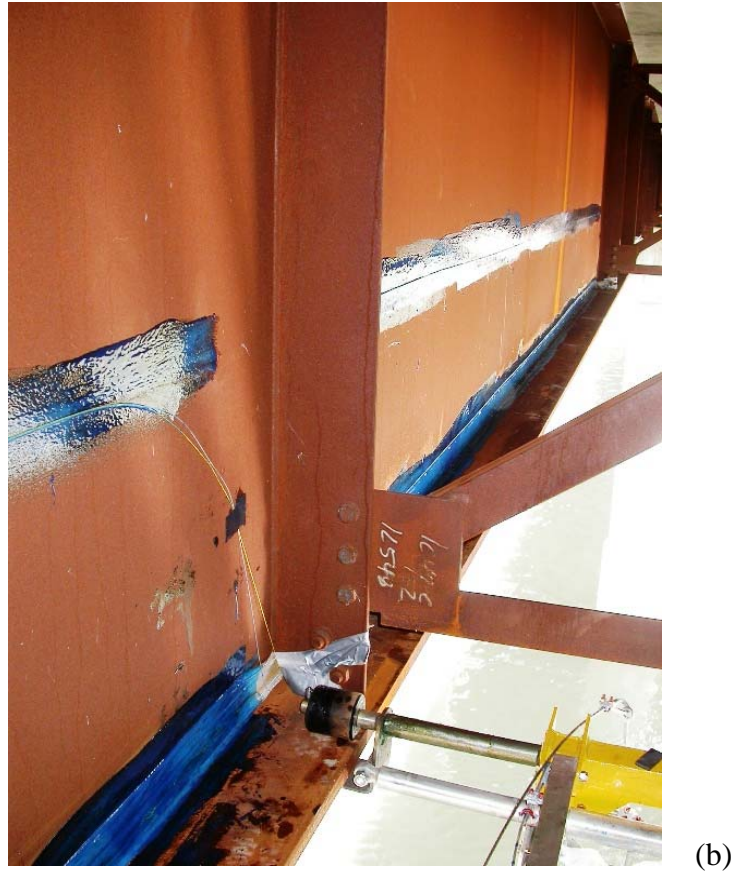
Figure 13 – Strain gauge measurements on Girder 2 at Location II: (a) comparison with Girder 1 at Passes A, B and D; and (b) photograph of FOS arrangement.
