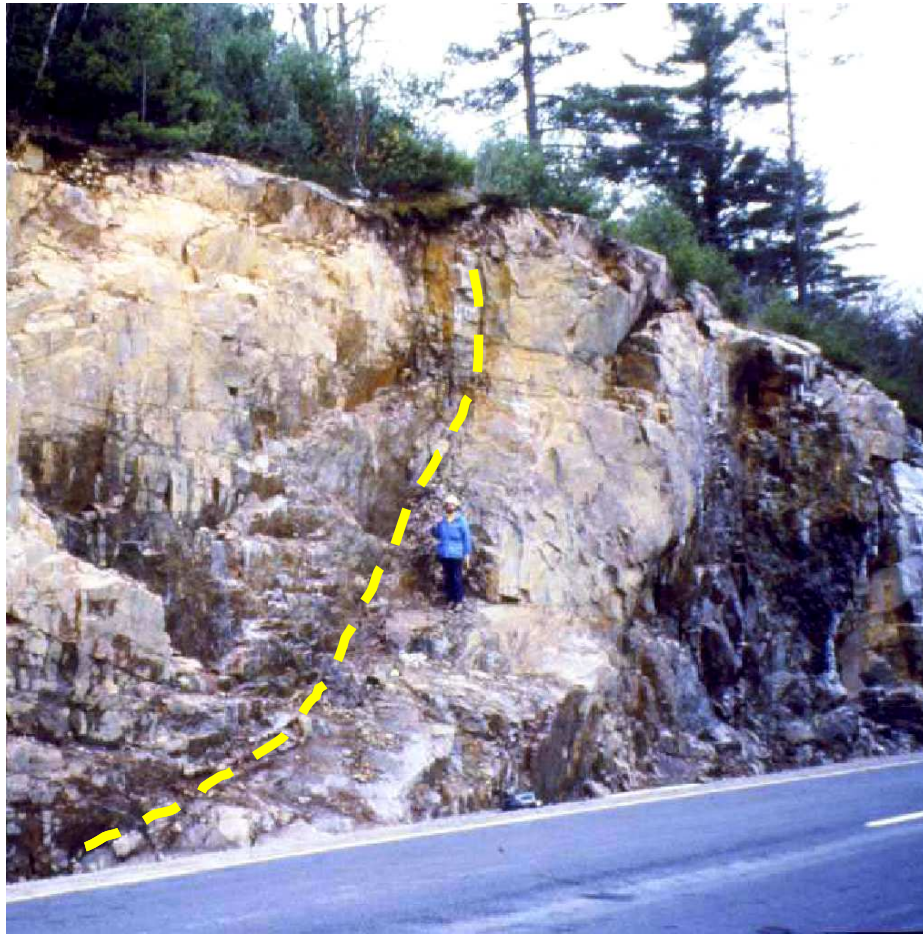
Figure 1.2: A rock failure along a hidden sub-vertical joint resulting in the death of a truck driver on Highway 401, Brockville, Ontario, Canada. Dr. Norbert Maerz, the advisor of this research, is standing beside the sub-vertical joint trace after removal the failed materials (dashed yellow line) (Adopted from Maerz and Kim, 2000).
