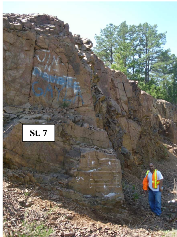
Figure 6.25: A front view of the rock slope of St.7 in site 2 (Madison County).
