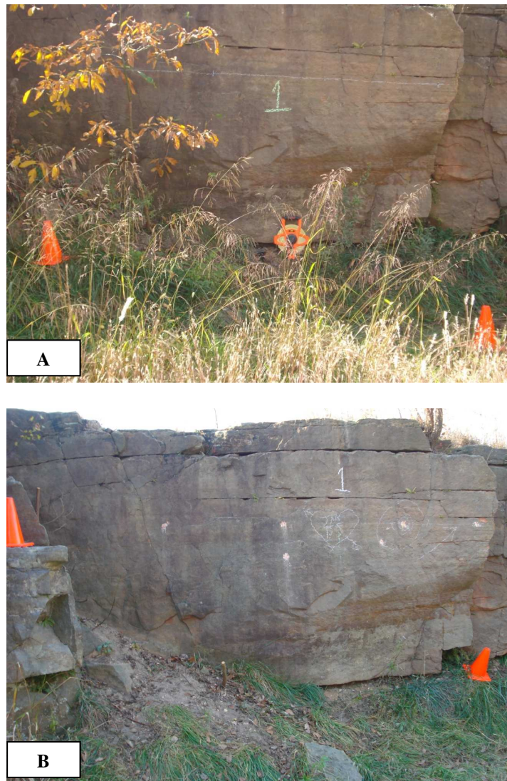
Figure 5.31: Station 1 before (A) and after (B), respectively, removing the grass to create a clean view for using the LIDAR. Notice that the locations of the three index.
