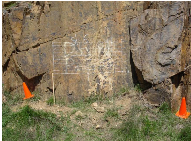
Figure 6.21: A front view of the rock slope of St.2 in site 2 (Madison County).
