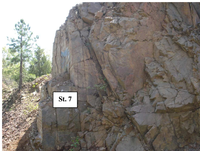
Figure 6.26: A side view of St.7 in site 2 is showing some discontinuities dipping steeply into the slope face which may cause toppling failure in the future (Madison County).
