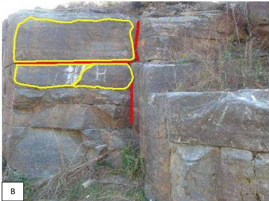
Figure 1.1: (A) A rock cut; (B) The same rock cut showing both joint traces (red lines) and facets (yellow polygons).
