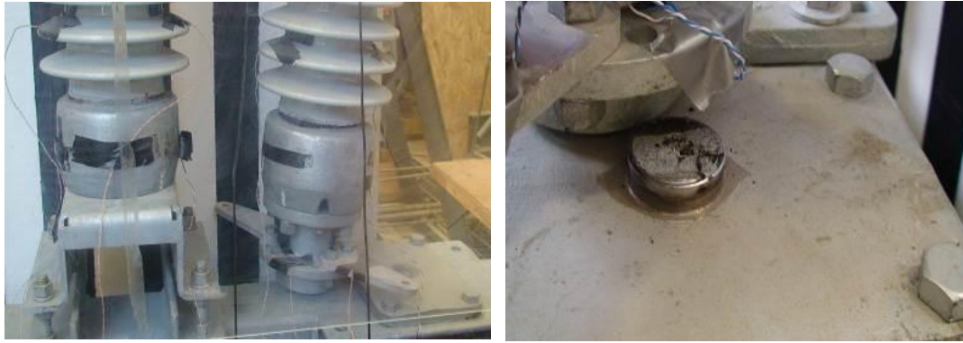
Figure 7.14. Fracture Detail and Failure Location
