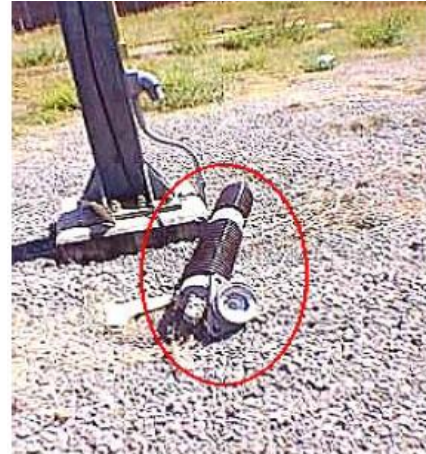
(b) Broken Bushing of a lightning rod
