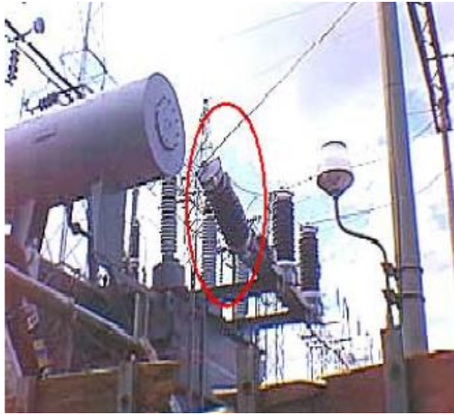
(a) Broken Bushing of a Transformer
