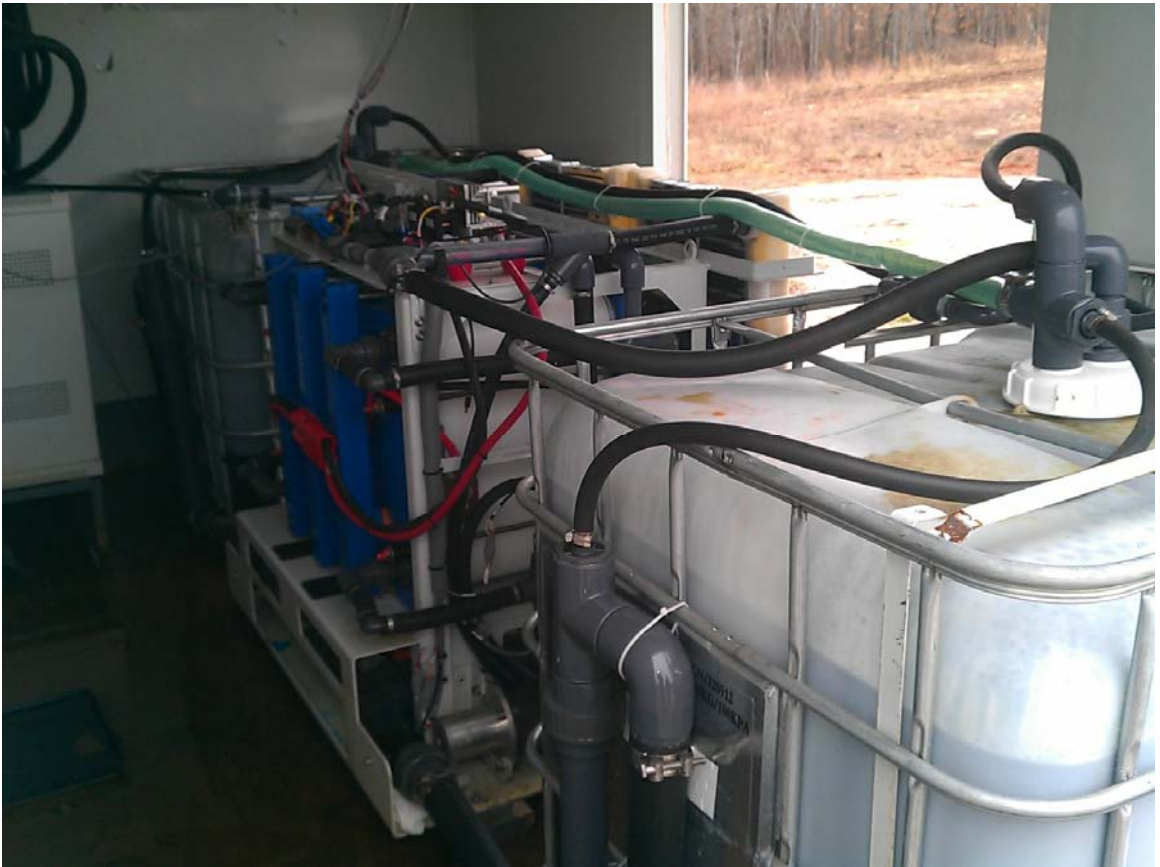
Figure A.4. VRB electrolyte tanks and stack
