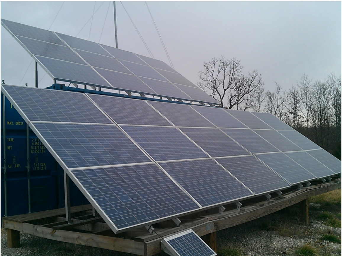
Figure A.2 PV array mounted on main container
