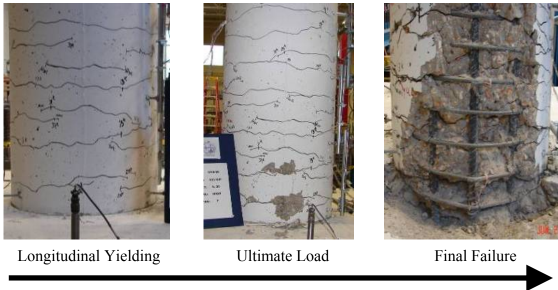
Figure 4.4 Damage to Column H/D(6)-T/M (0.0)-0.73% under Flexure
