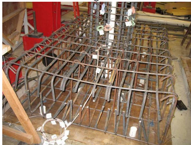
Figure A.4 Column Sectional Detail and Photo of Foundation Reinforcement (All dimensions in inches, 1 inch= 25.4 mm)
