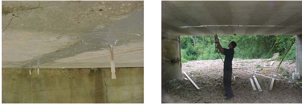
(a) Crack sealed prior to injection (b) Crack injection underneath the bridge
