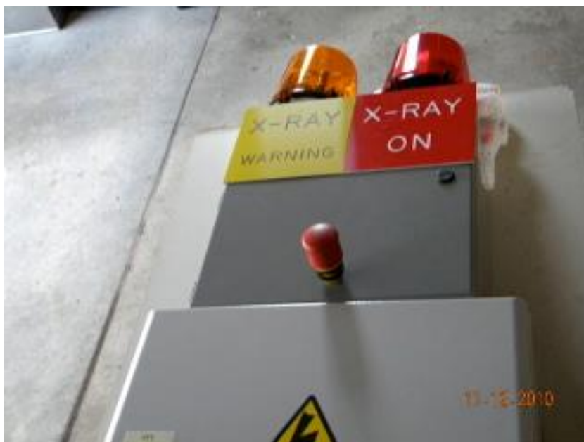
Figure A.5. Radiation Safety Alarm and Direct Disconnect Switch
