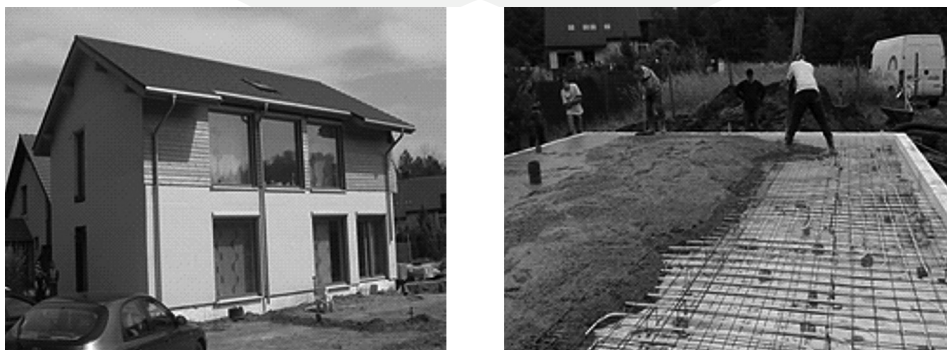
Fig. 1. Passive house in Boruszowice (left) and slab on grade during construction (right)
