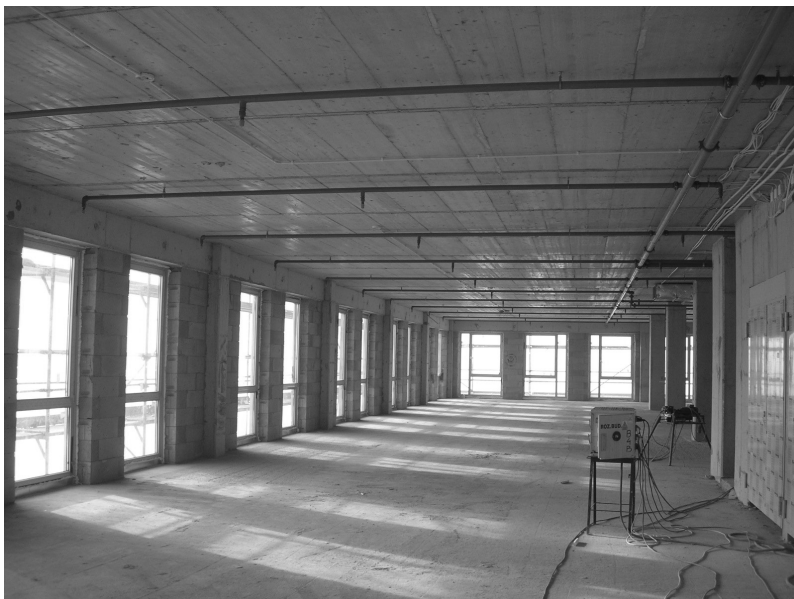
II. 3. Shell and Core office building – before the interior was arranged by the tenant (Photo from the archive of the Artur Jasiński i Wspólnicy design office)
