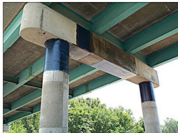
Fig. 7. Fiber-optic sensors installed on the reconstructed pier cap of an I-44 overpass. The crack sensors and the patch box are visible on the face and the delamination sensors are placed on the blue reinforcing sheet on the bottom.
