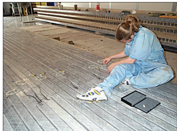
Fig. 4. Fiber-optic sensors are embedded in the bottom layer of the smart composite bridge during assembly. The full-scale I-beam test article is shown in the background.
