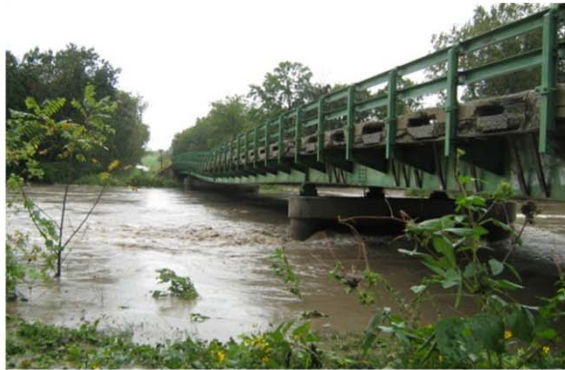
(a) Loss of center pier
