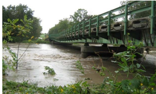
Figure 1.1 Loss of a Center Pier of the Thompson River Bridge, Missouri
