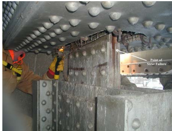
Figure 1.4 Point of Strut Failure
