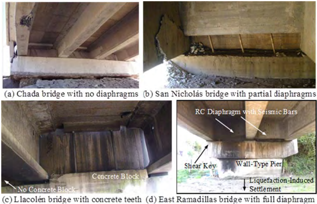
Fig. 1.1 Observed performance of highway bridges during the 2010 Chile Earthquake.
