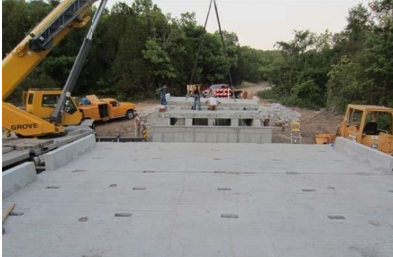
Figure 5.12: Completion of all concrete deck slabs on top of steel- and concrete- girders
