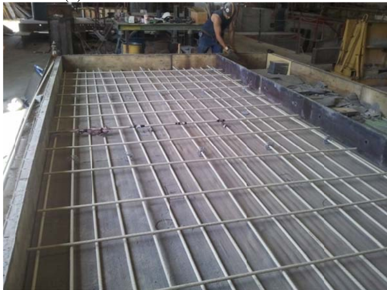
(b) Top layer of reinforcement (casting upside down of the precast slab)
