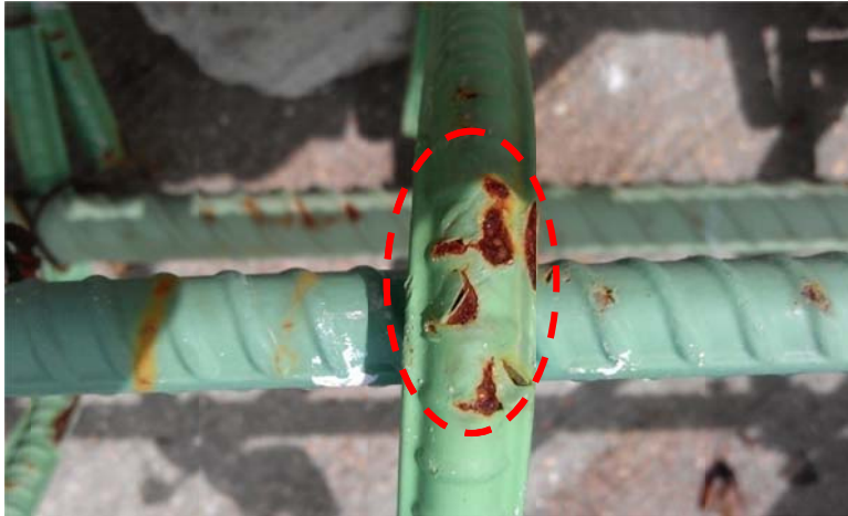
Figure 2.3: Damaged epoxy coating and rebar corrosion
