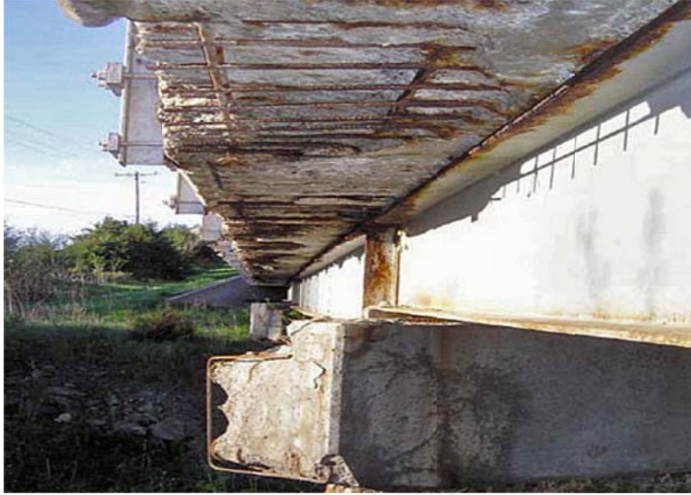
Figure 2.1: Missouri deteriorated bridge deck (from the Missouri Department of Transportation in http://minnesota.publicradio.org/display/web/2008/02/11/missouri_bridges/ )
