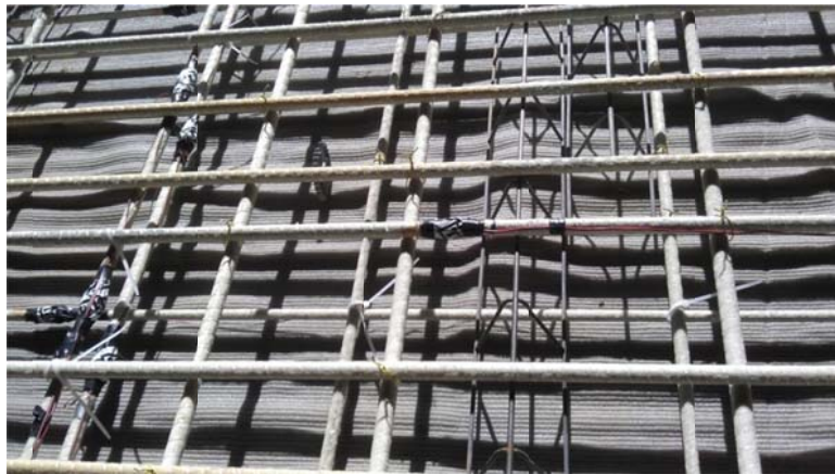
Figure 5.6: Strain sensors in concrete deck slab
