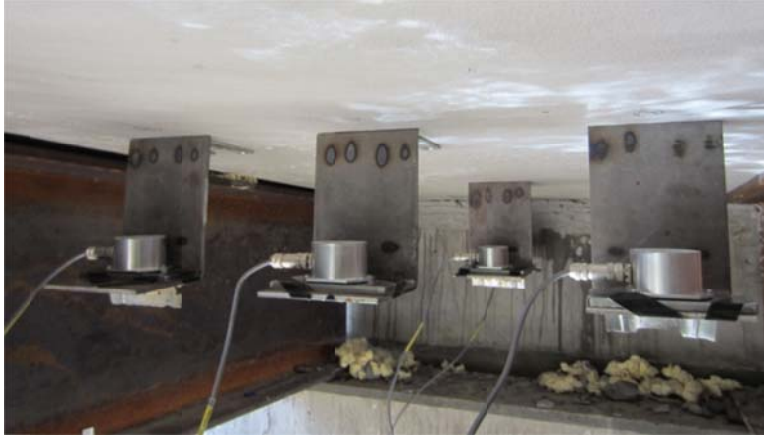
(a) Steel-girder span (6 inclinometers)
